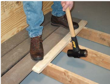
Set next course of decking by driving onto "claws" with long handle sledge hammer.
